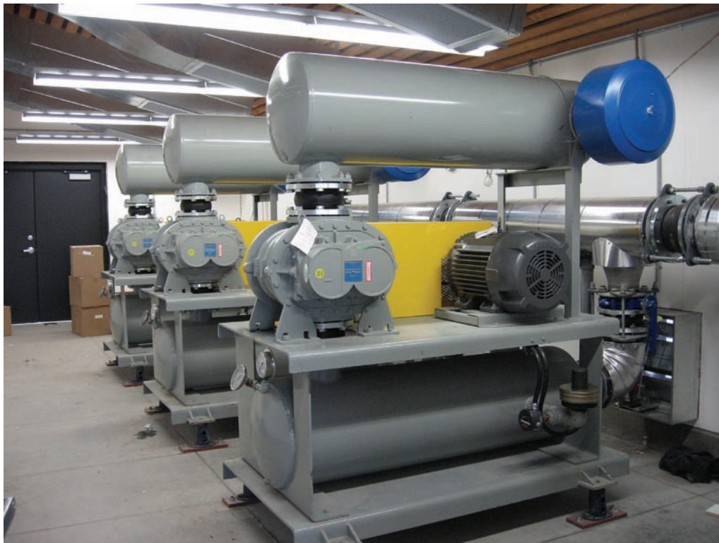
Lagoon Aeration Blowers
