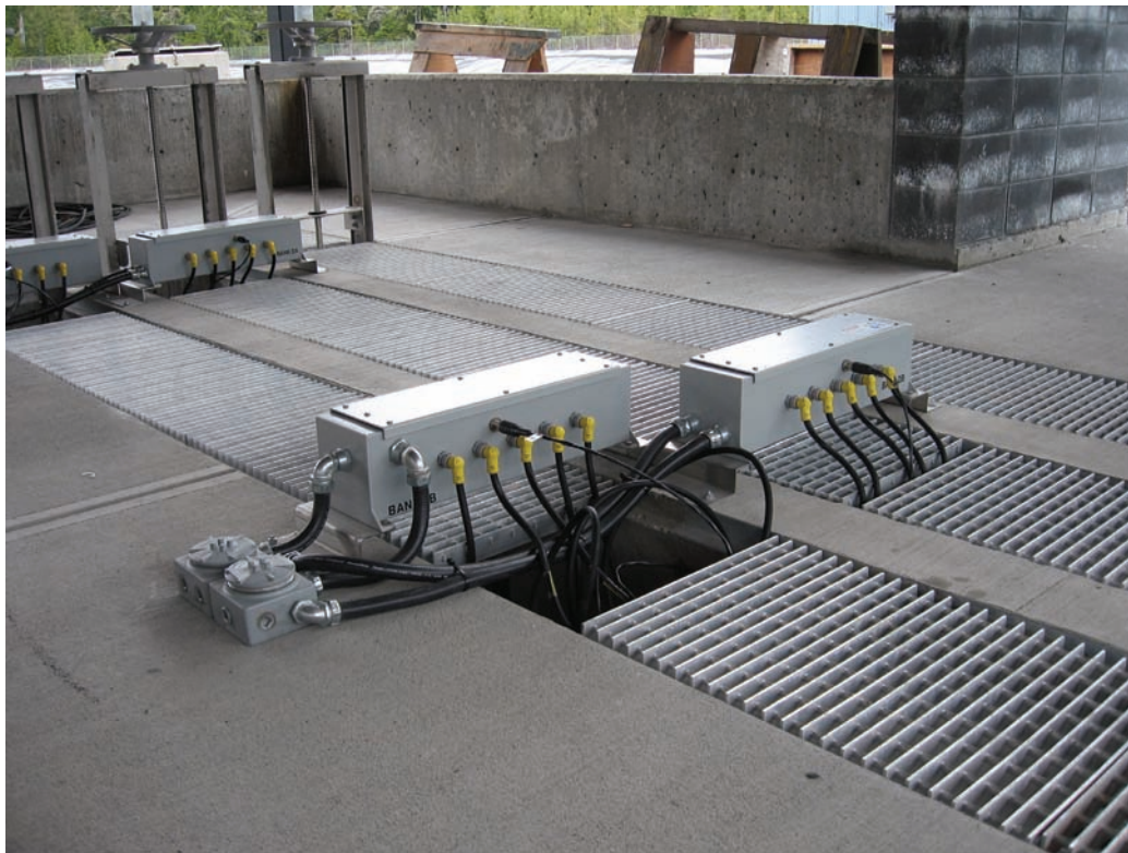
UV Disinfection at Lagoon Outlet
