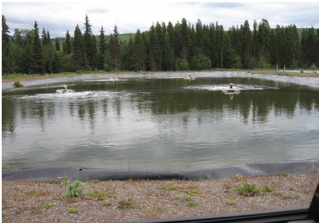
Lagoon Surface Aerators
