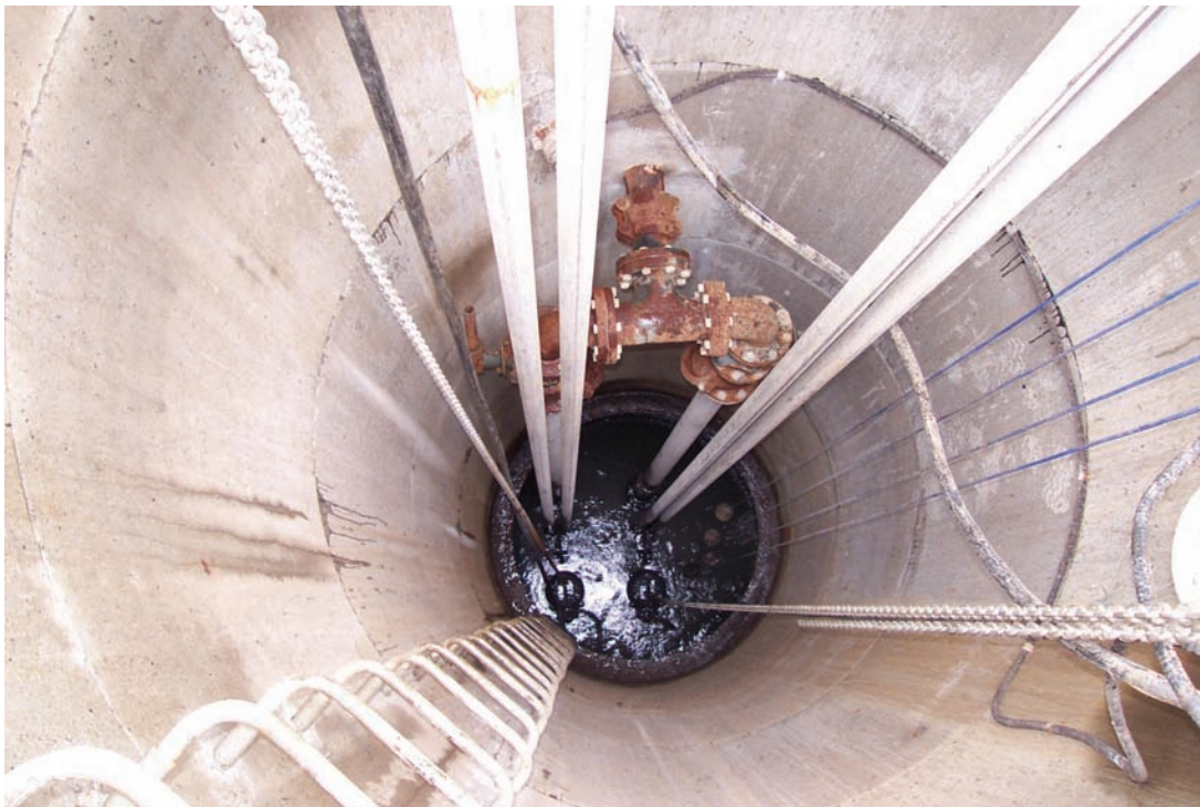
Inside of Pump Station
