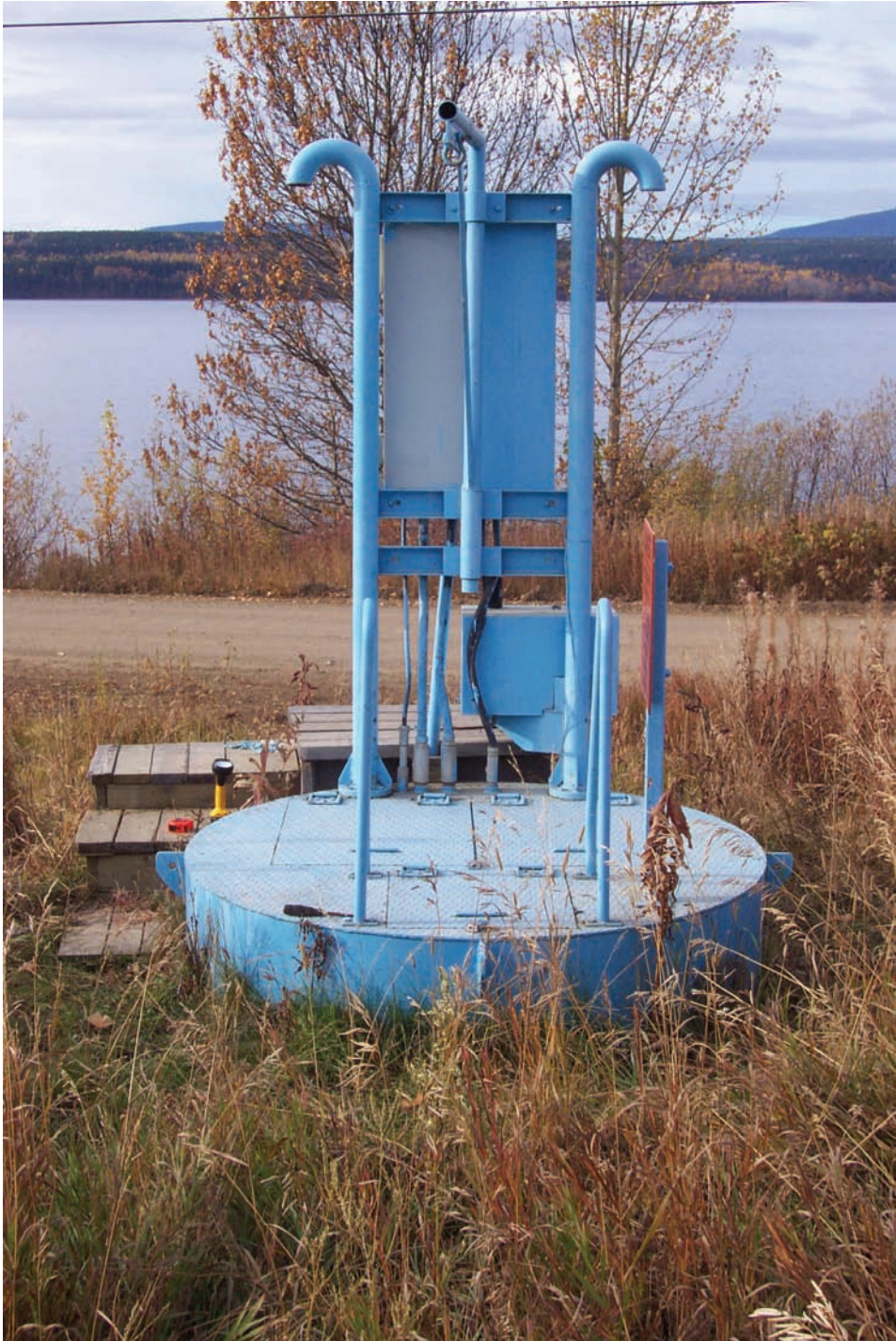
Submersible Pump Station
